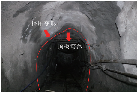
图 8 巷道变形破坏状况 Fig.8 Failure state of the roadway
